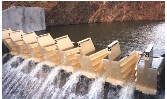
SLIGHT OVERSPILLING ABOVE THE FUSEGATES CREST AT MCCLURE DAM, NEW MEXICO
