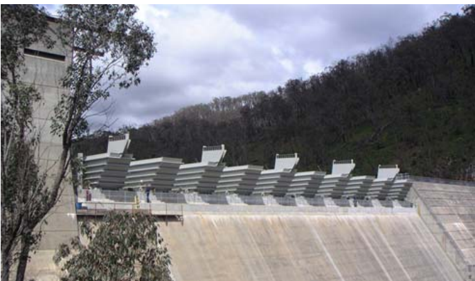
FUSEGATES ONTO SPILLWAY
